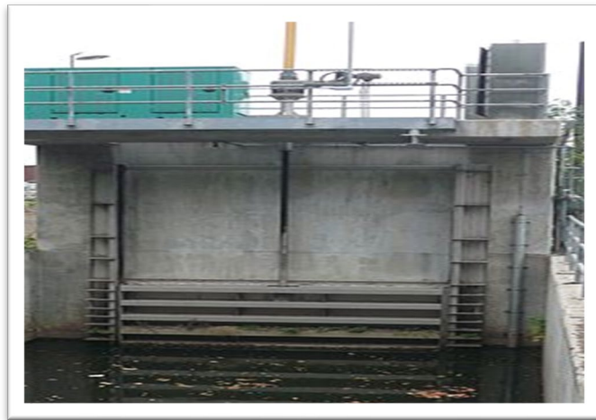
Hydraulic Sluice Gate
