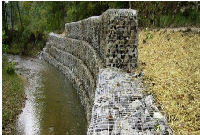
Rajah 5.3.i Gabion Mattress
