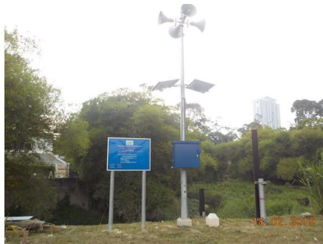
Rajah 4.2.3.ii Stesen siren di Hulu Langat, Selangor.
