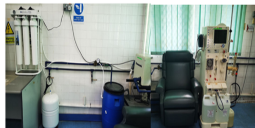
Figure 6: The RO System - Tank for Hemodialysis (HD) Running System
