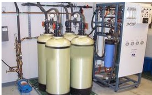
Figure 2: The sample of real RO system-Tank for HD system at the hospital
