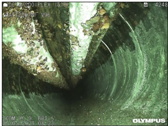
Fig. 1 A look inside the guard. UngROUTED guard, visible subsidence of the grouting material. Corrosion of prestressing reinforcement wires
