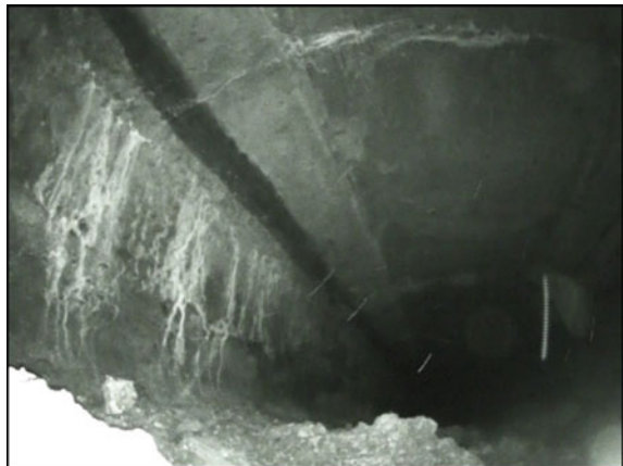
Fig. 2 A look inside the KA girder's chamber. Visible active leak traces. Corrosion of the exposed reinforcement
