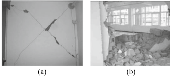
Fig. 4 (a) Example 1 of infill wall damage (b) Example 2 of infill wall damage
