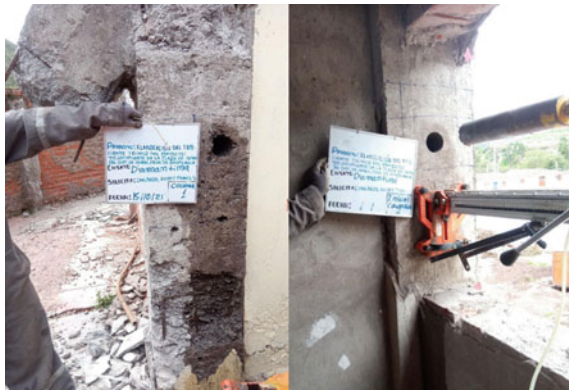
Fig. 5 Removal of concrete cores on the first and second levels of the clock tower
