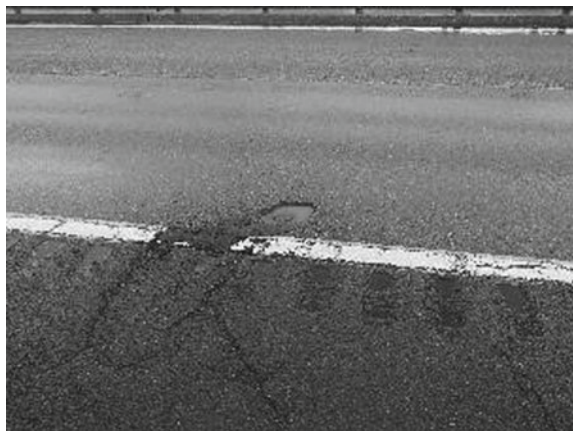
Fig. 1 Potholes and cracks on the road surface
