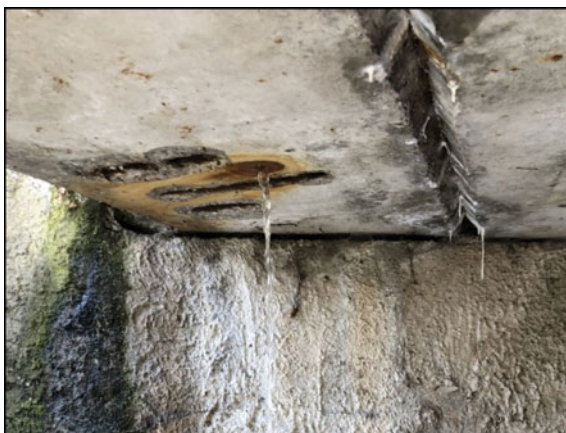
Fig. 3 View of the bottom face of the KA girders. The chambers of the girders were flooded with water due to malfunctioning waterproofing
