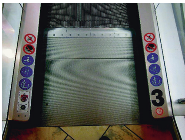
Fig. 28.26 Comb plate with comb segments at the lower landing station. (source: author)
