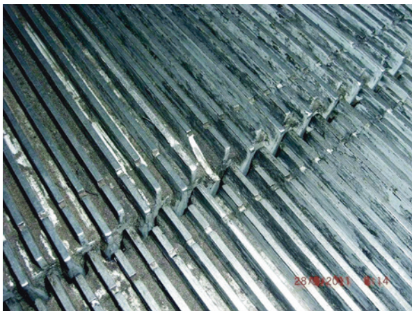
Fig. 32.5 Broken web on an escalator step. (Source: Author)
