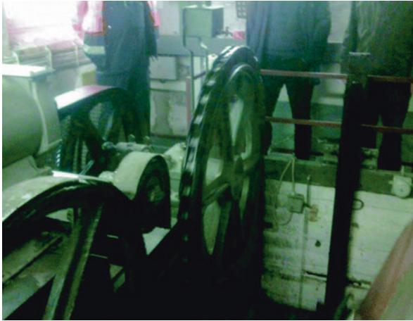
Fig. 4.11 Diverter pulley in the engine room of a paternoster. (Source: Author)
