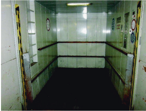
Fig. 4.2 View of a freight lift car with safety light grid. (Source: Author)
