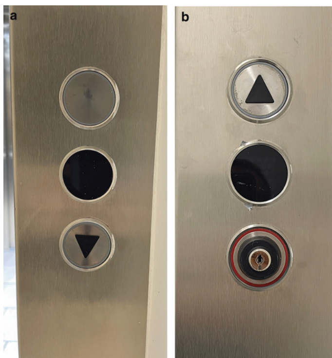
Fig. 7.9 a + b External call panels at the terminal stops (Source: Author)
