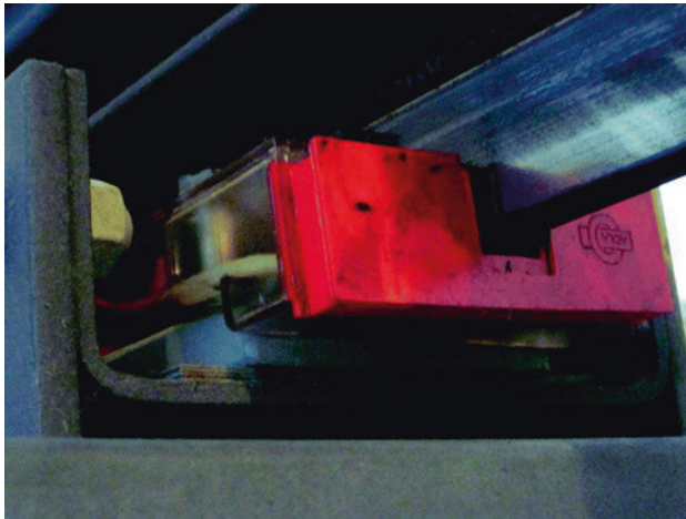
Fig. 5.9 Rail oiler on the car roof for lubricating the guide rails. System with sliding guide. (Source: Author)
