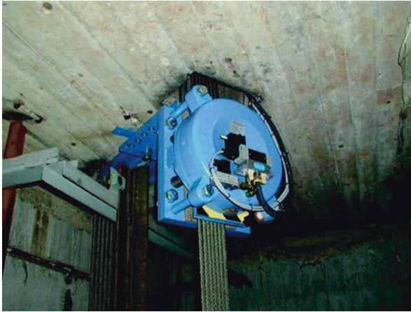
Fig. 13.4 Rope brake installed under the well head ceiling. (Source: Bode Components GmbH, Düsseldorf)
