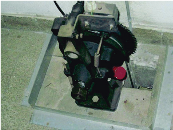
Fig. 10.3 Overspeed governor of an older system built around 1965. (Source: Author)
